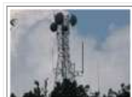
Antennas atop the "FAAT" facility
